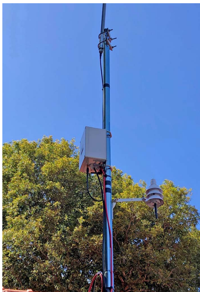
The input module, installed next to the controller, is wired in and connected to the point-to-point transmitter mounted in open air space.
